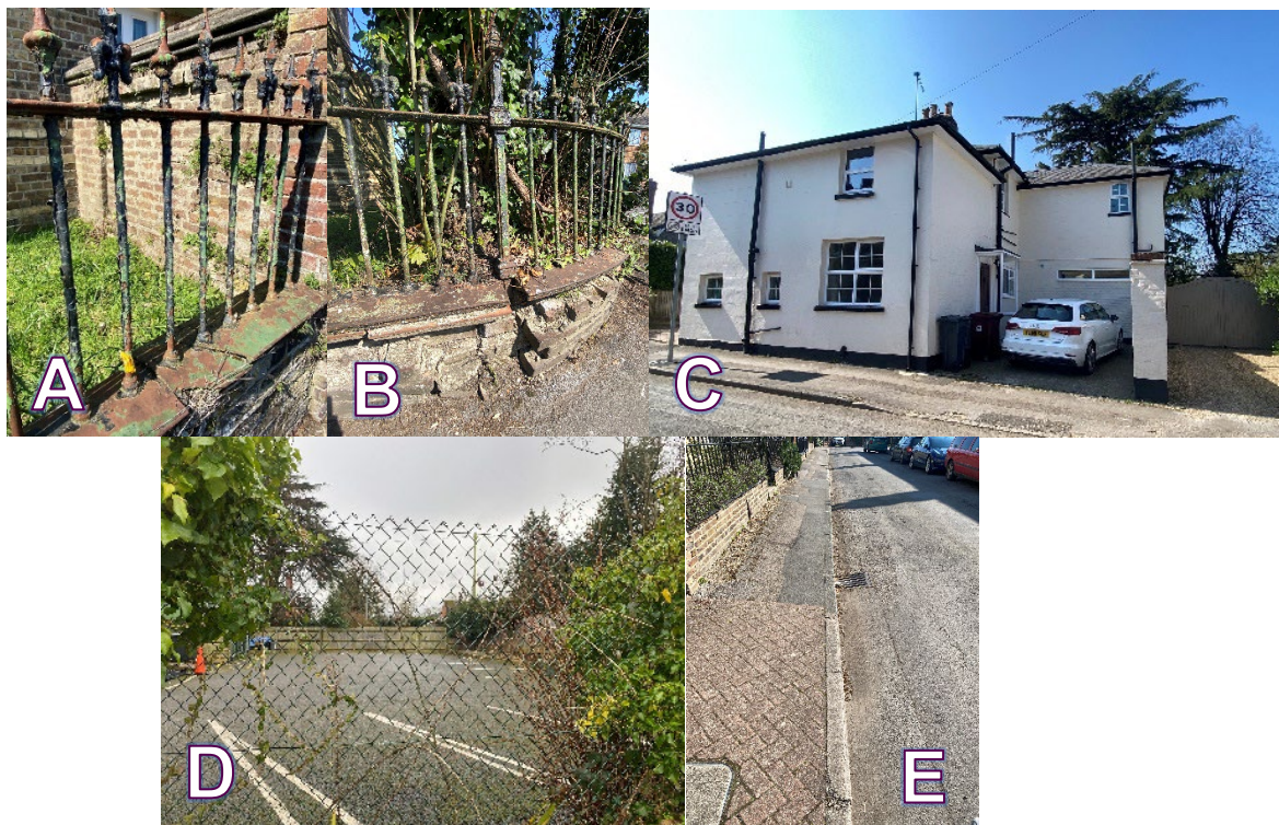
Figure 26: Images of loss or deterioration of details (Images Claire Truman)
