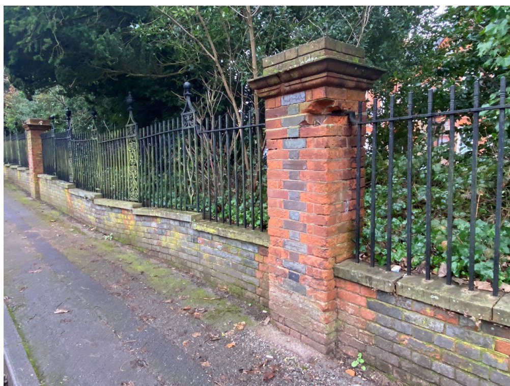
Figure 22: The brick piers and railings to Hillside are falling into disrepair – view along Lower Mount (Image Claire Truman)
